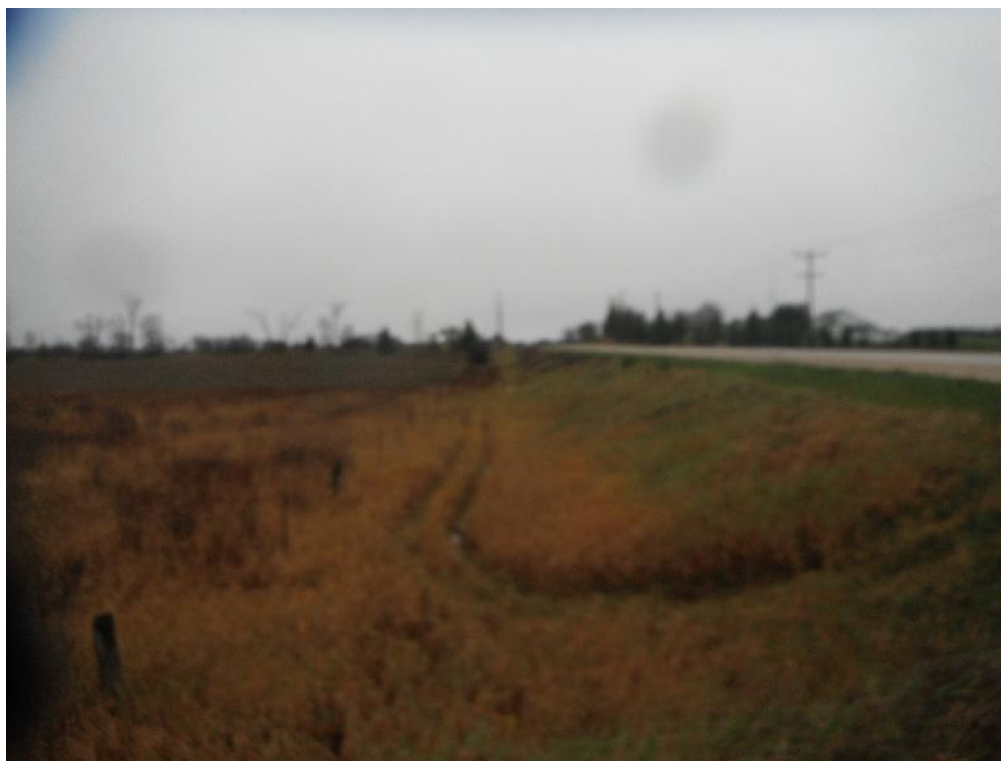
Plate 12: Change in access road area, slope from Grey Road 4 with poorly drained area at base (Figure 4), facing east
