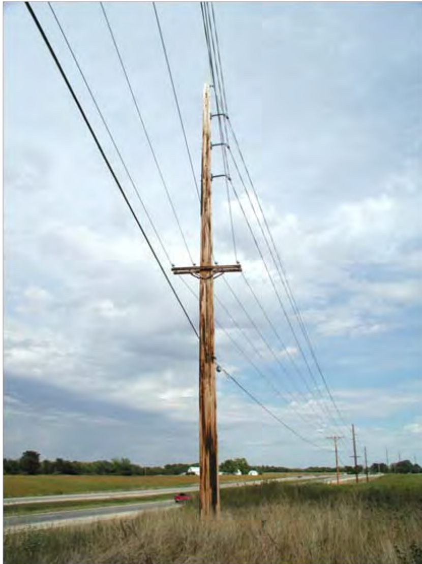
Figure 3: Example of joint use or pole sharing
