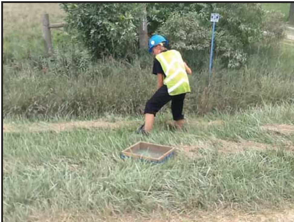
Image 214: View of Crewmember Test Pitting to Confirm Disturbance at Mollard Line from GSH1559 to GSH1099 (Photo Taken August 26, 2013; Facing East)
