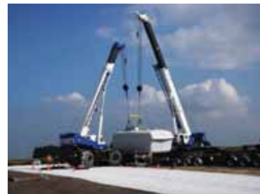
A wind turbine component, known as a nacelle, is lifted from a truck.
