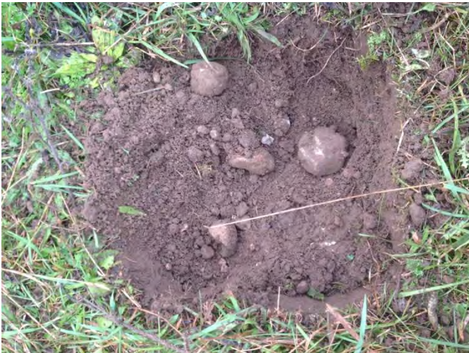
Plate 27: Study area 7, EDU 1008, example of disturbed test pit from mounded areas; view west
