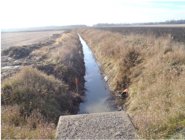
Photo 3 Station 16-1 – Elliot Drain (Fall 2011) - Facing upstream (south) from Townsend Line showing culvert and recently cleared channel.
