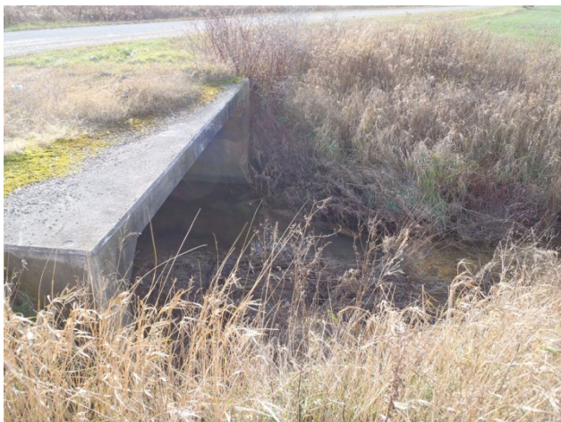
Photo 5 Station 11-1 – Woods Creek (Fall 2011) – Facing west along Cedar Point Line showing close-up of culvert.
