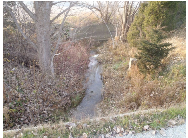
Photo 4 Station 18-1 – Douglas Drain (Fall 2011) - Facing downstream (west) from Hillsboro Road showing culvert and channel overview. Note the concrete deflection wall in the background.
