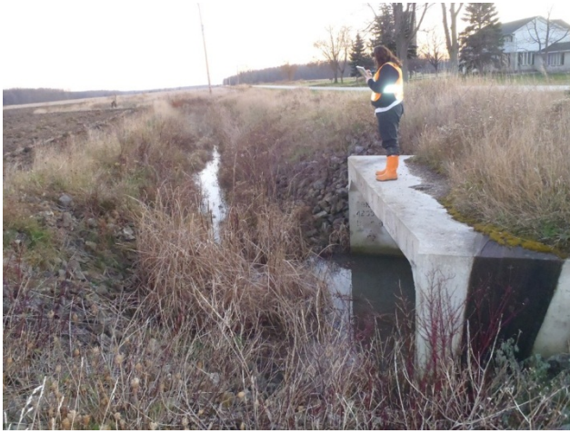
Photo 13 Station 34-2 – Bannister Drain (Fall 2011) - Facing upstream (south) along the east side of Hillsboro Road showing culvert and channel overview.
