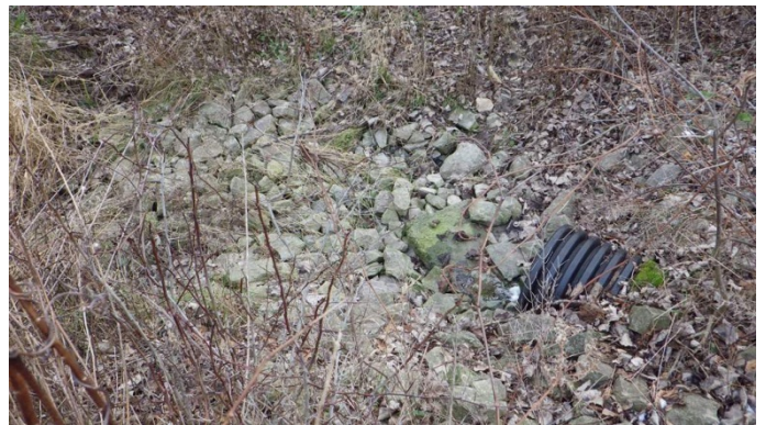
Photo 6 Station 53-5 – Mud Creek-1 (Summer 2012) – Showing outlet of piped/tiled watercourse under Mud Creek-1, outlets into floodplain of Mud Creek.
