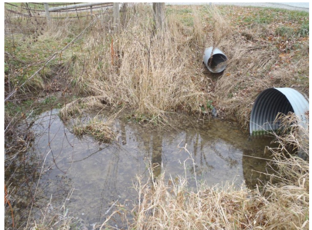
Photo 34 Station 22-2 – Unknown Drain (Fall 2011) - Close-up of upstream culvert showing large pool and roadside drainage inputs.
