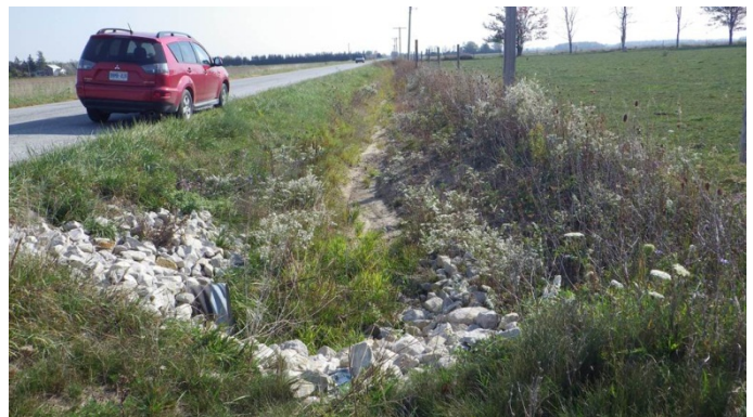
Photo 18 Station 19-3 – Unknown Drain 2 (Fall 2012) – Facing upstream (east) showing incised channel along south side of Hubbard Line.
