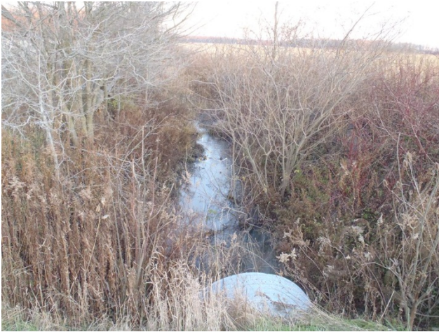
Photo 9 Station 34-1 – Watson Drain (Fall 2011) - Facing upstream (east) from Hillsboro Road showing culvert and channel overview.
