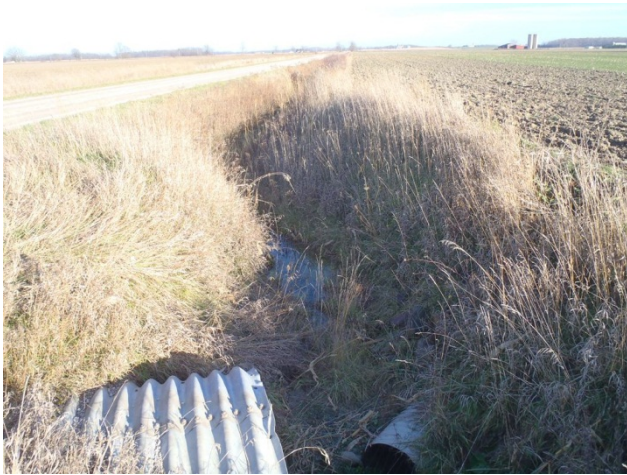
Photo 13 Station 5-1 – Beith Creek Drain (Fall 2011) – Facing upstream (east) along Proof Line showing culvert, tile drainage inputs and channel overview.
