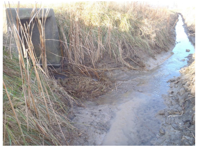
Photo 4 Station 16-1 – Elliot Drain (Fall 2011) - Facing downstream (west) from roadside ditch show culvert and channel.
