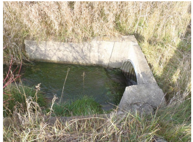
Photo 16 Station 20-2 – Fisher Drain (Fall 2011) - Close-up of upstream algae lined culvert.
