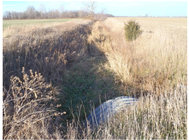
Photo 14 Station 5-1 – Beith Creek Drain (Fall 2011) – Facing downstream (north) from Proof Line showing culvert and channel overview. Note the watercress in the foreground.
