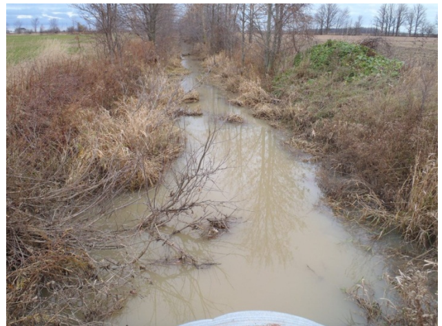
Photo 6 Station 2-2 – Lusby Drain (Fall 2011) - Facing downstream (north) from farm crossing showing culvert and channel overview.
