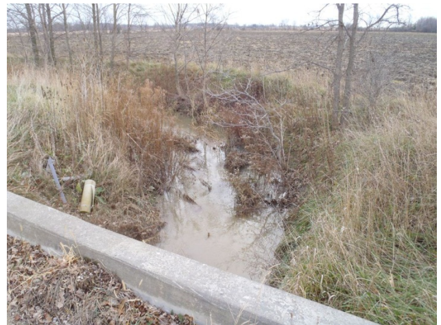
Photo 16 Station 4-1 – Ross Drain (Fall 2011) - Facing downstream (north) from Thomson Line showing culvert and channel overview.
