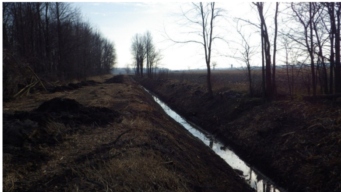
Photo 21 Station 4-5 – Stewardson Drain (Fall 2012) – Facing upstream showing recently cleared channel.
