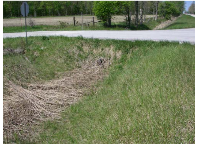
Photo 2 Station 16-5 – Anderson Drain (Spring 2012) – Facing downstream (northwest) along Townsend Line showing cattail lined channel.
