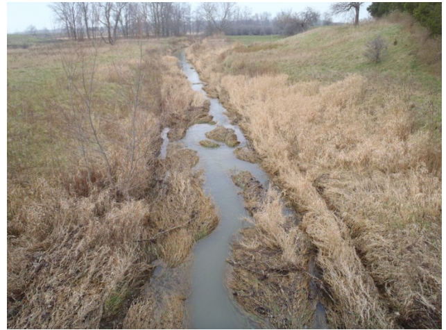
Photo 2 Station 31-3 – Highland Creek (Fall 2011) - Facing downstream (north) from Douglas Line showing braided flow through grass lined channel.
