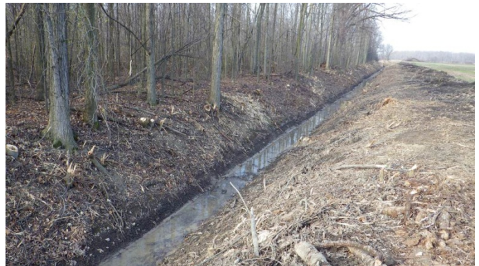
Photo 22 Station 4-5 – Stewardson Drain (Fall 2012) – Facing downstream showing incised channel.
