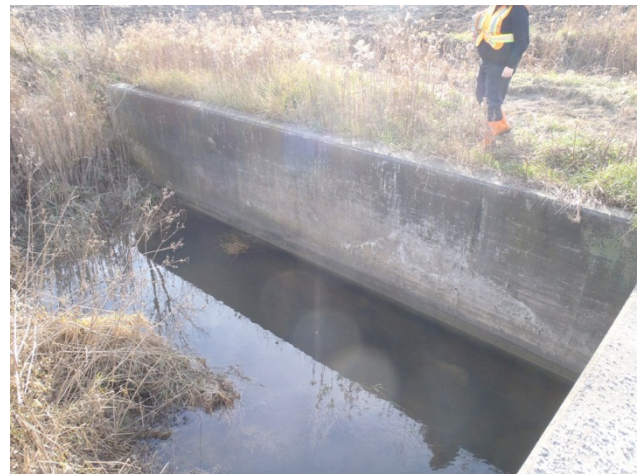
Photo 4 Station 11-1 – Woods Creek (Fall 2011) - Close-up of upstream culvert and deflection wall to divert westerly flow north.
