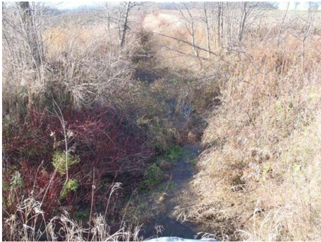
Photo 19 Station 12-2 – Brush Drain (Fall 2011) - Facing downstream (west) from Fuller Road showing culvert and channel overview. Note the patch of watercress downstream of the culvert.
