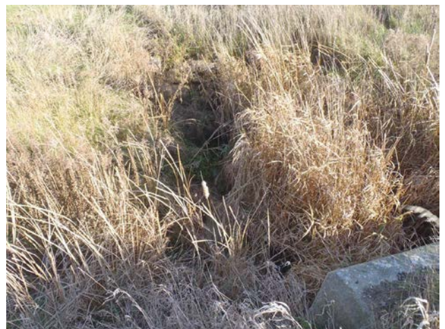
Photo 6 Station 6-1 – Wadsworth Drain (Fall 2011) - Facing upstream (east) from Rawlings Road showing culvert and surrounding vegetation.
