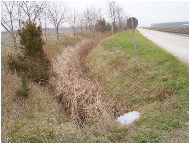
Photo 15 Station 31-1 – Hartley Drain (Fall 2011) - Facing upstream (south) along the east side of Hillsboro Road showing channel densely lined with cattails.
