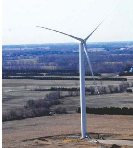
First GE 2.5 MW turbine in North America - Kent Breeze Wind Power Project
