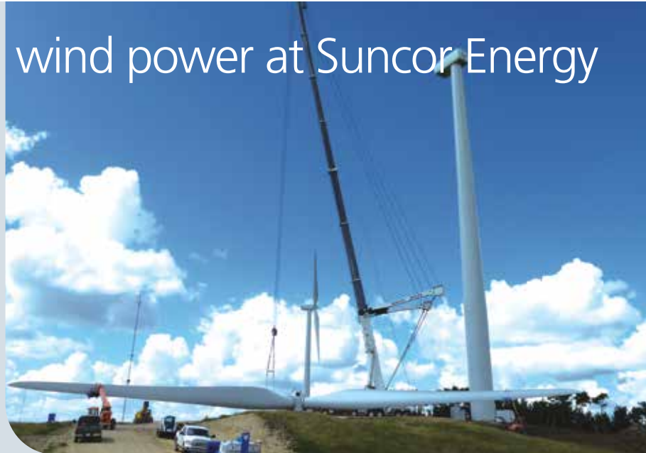
Lifting a 47.5-tonne rotor assembly into the air and onto the nacelle of a turbine.
