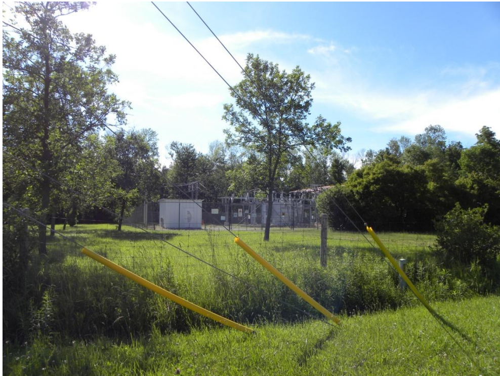
Plate 4: Transformer Station, south of Townsend Line on Elarton Road, looking west.
