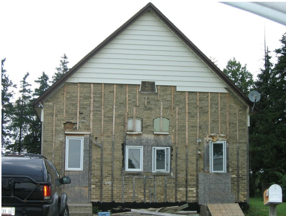
Plate 14: S. S. No. 10 Plympton, located at northwest corner of the intersection of Michigan Line and Oil Heritage Road. Currently in use as a residence.
