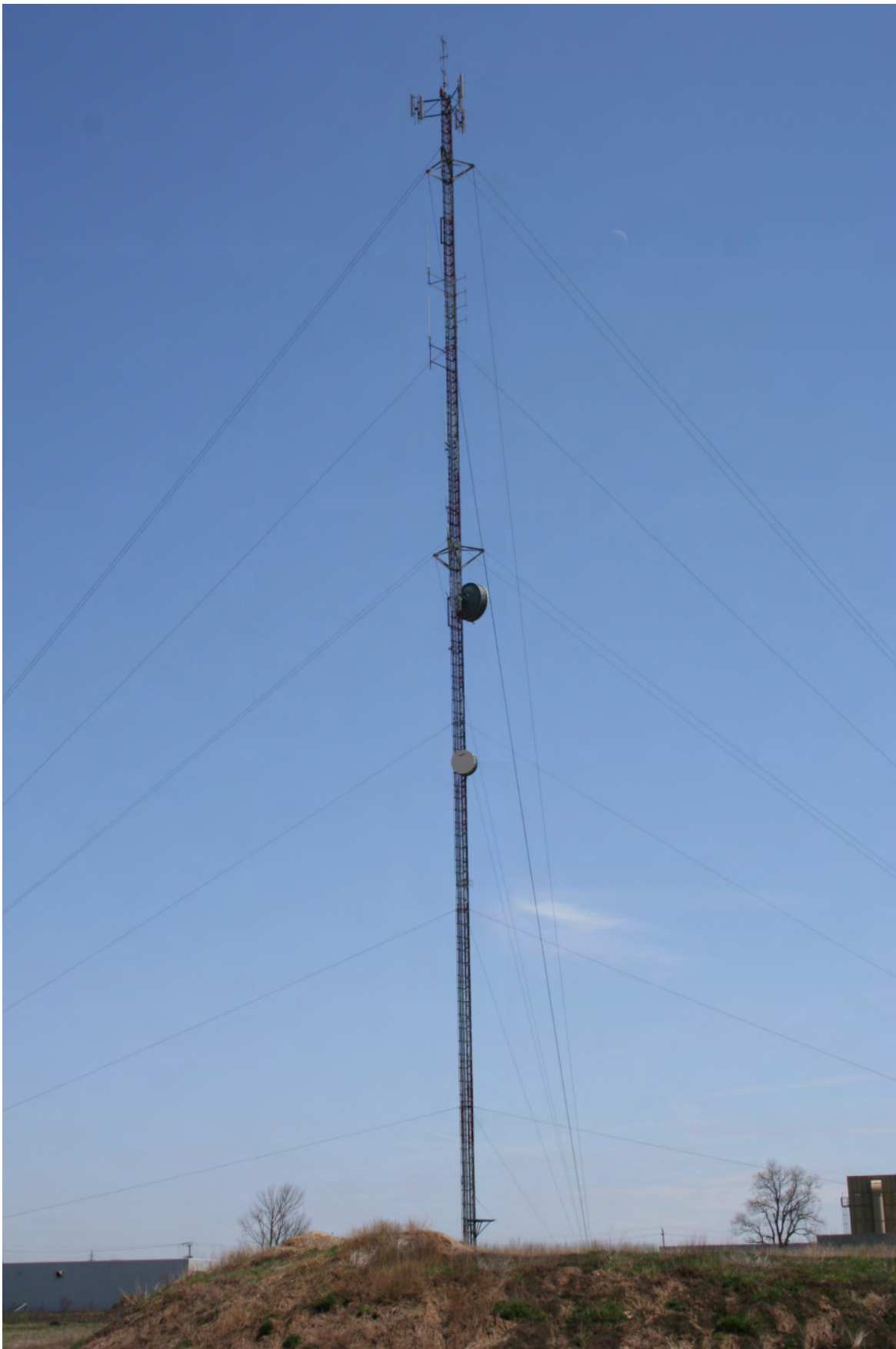
STRATHROY TELECOM TOWER ON HIGHWAY 81 BEHIND MOTEL AT 2ND STREET. TAKEN FROM HIGHWAY 81 LOOKING EAST BEHIND MOTEL
